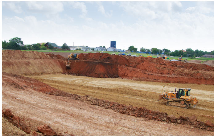
The process of digging the foundation and basement for the new Immaculata project in St. Marys, KS was a monumental task.
