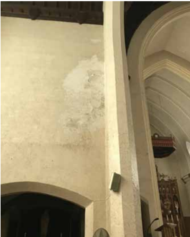
Before: Damaged walls and sanctuary.
