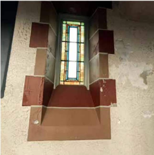
Before: Painted quoining around small stained glass windows inside the church.
